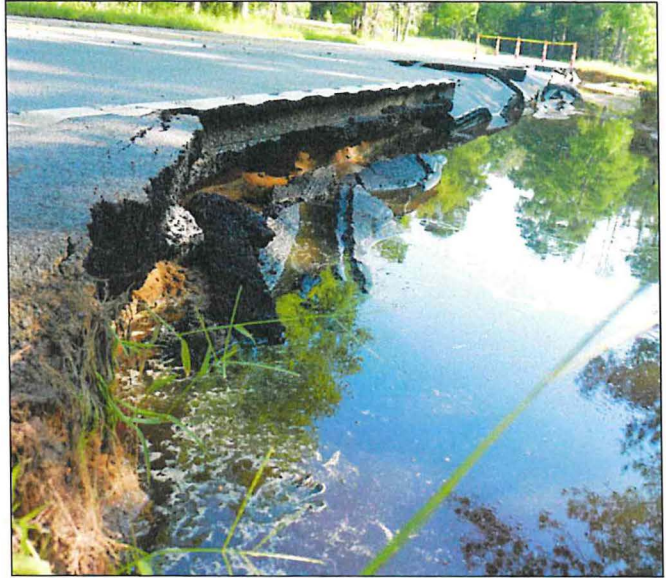
Photos of the road washed out on State Park Road, near Blow Horn Place. Photos By Landry Collins/The Dillon Herald
